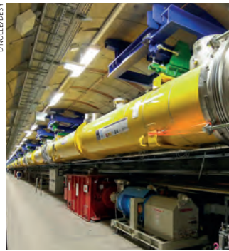
The main accelerator tunnel of the European XFEL.
